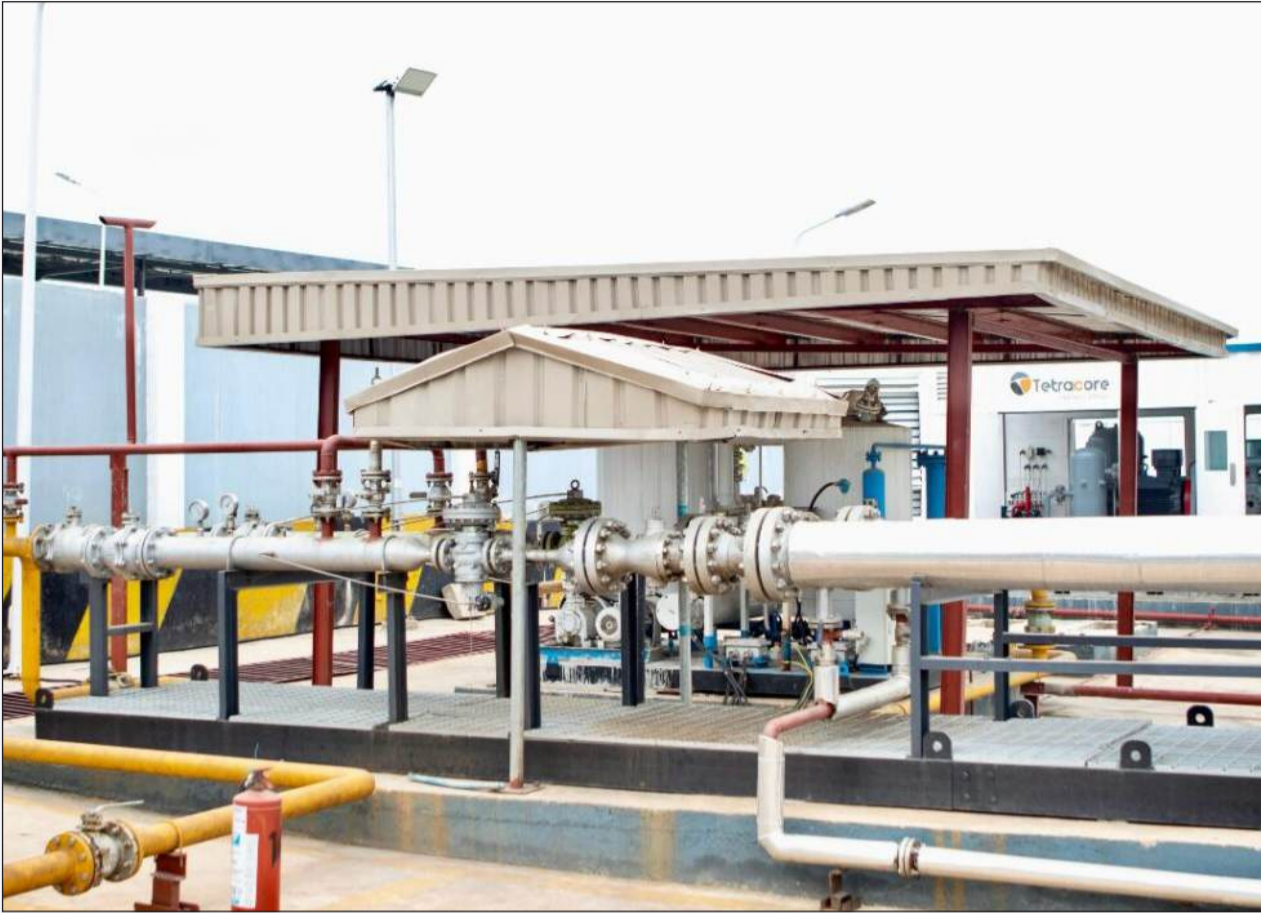
Tetracore's Atakobo Industrial Park (CNG FACILITY) in Ogun State, with a capacity of 6.2 MMscf/d
