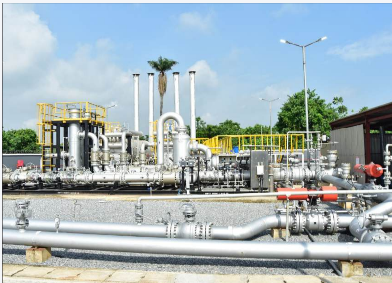
Axxela's natural gas city gate facility in Ibe fun, Ogun state
