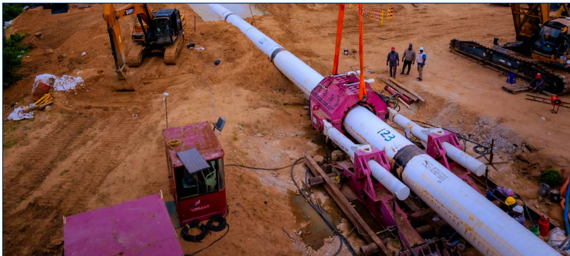
NNPC Limited Records Major Breakthrough with Successful River Niger Crossing on OB3 Gas Pipeline. The OB3 Pipeline is a strategic infrastructure designed to transport up to 2 billion standard cubic feet of gas per day - a backbone gas infrastructure linking the Eastern gas network to the Western network and extending connectivity to the Northern corridor through the AKK Pipeline.
