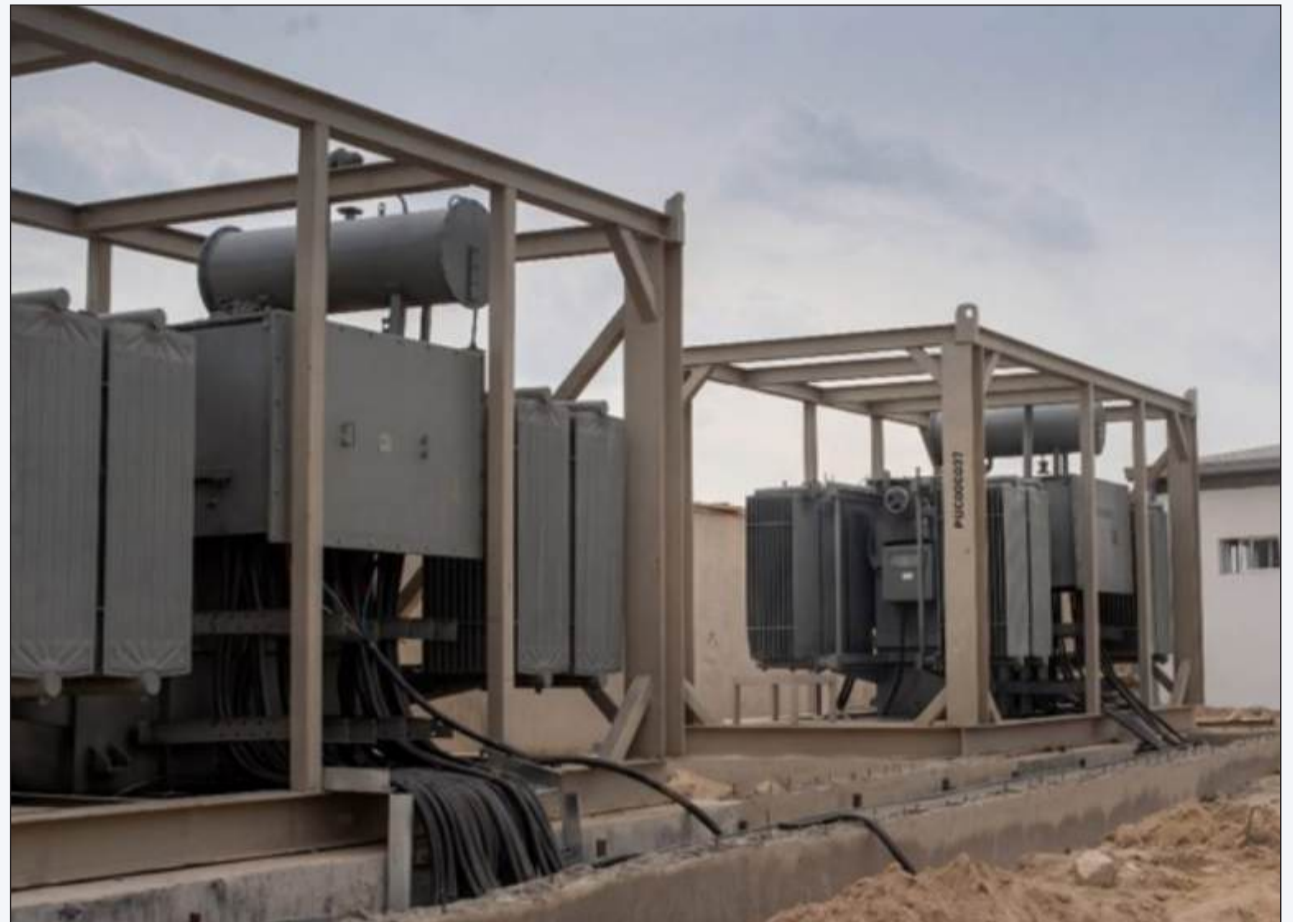
Tetracore's 100MW Atakobo Independent Power Generation & Distribution System
